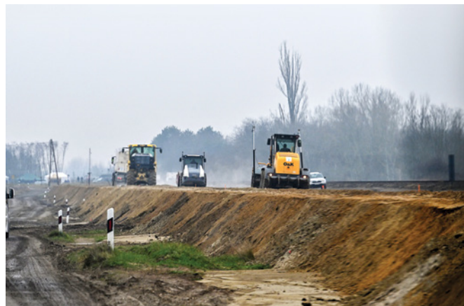
Construction vehicles prepare the bed for the Budapest-Belgrade railway line near the Hungarian-Serbian border in 2022. The 350-kilometer high-speed rail project, being built by a Hungarian-Chinese consortium, is part of China's economic investment in Central and Eastern Europe. AFP/GETTY IMAGES
