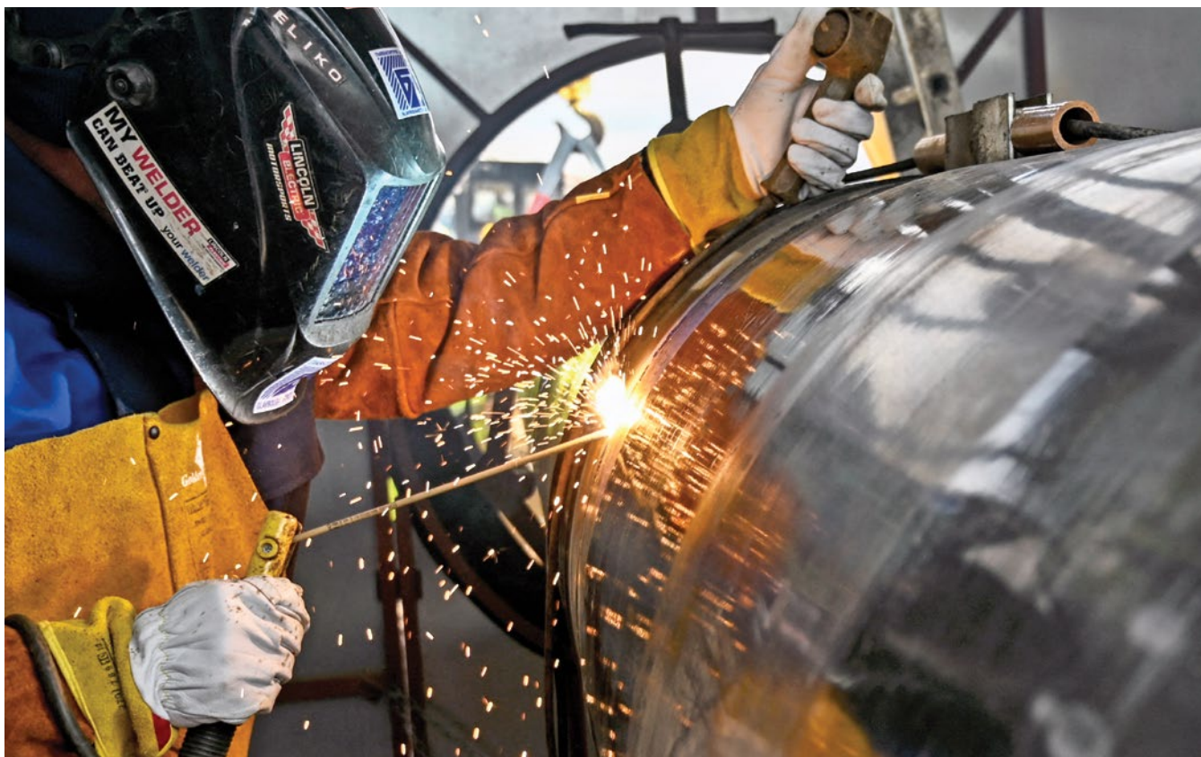
A worker welds a pipe on the Bulgaria-Serbia gas pipeline, near Kostinbrod, Bulgaria, in February 2023. The long-delayed connector pipeline will boost security of gas deliveries. AFP/GETTY IMAGES
