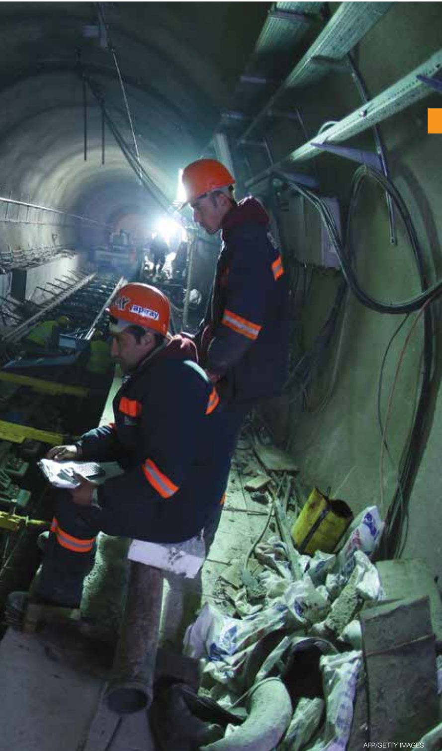
Turkish workers build a railway in the Marmaray Tunnel under the Bosphorus Strait in April 2013. The Marmaray project, which reflects Turkey's new economic confidence, includes the undersea tunnel and the modernization of suburban rail lines along the Sea of Marmara.
