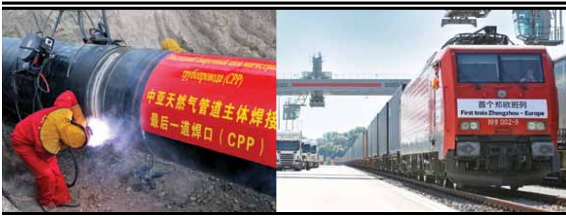
Workers weld the last links of Kazakhstan's segment of the Central Asia-China gas pipeline near Almaty in 2009.
